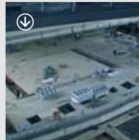
World's Largest Electric Stage Lifts Built to raise 20 elephants for international show
